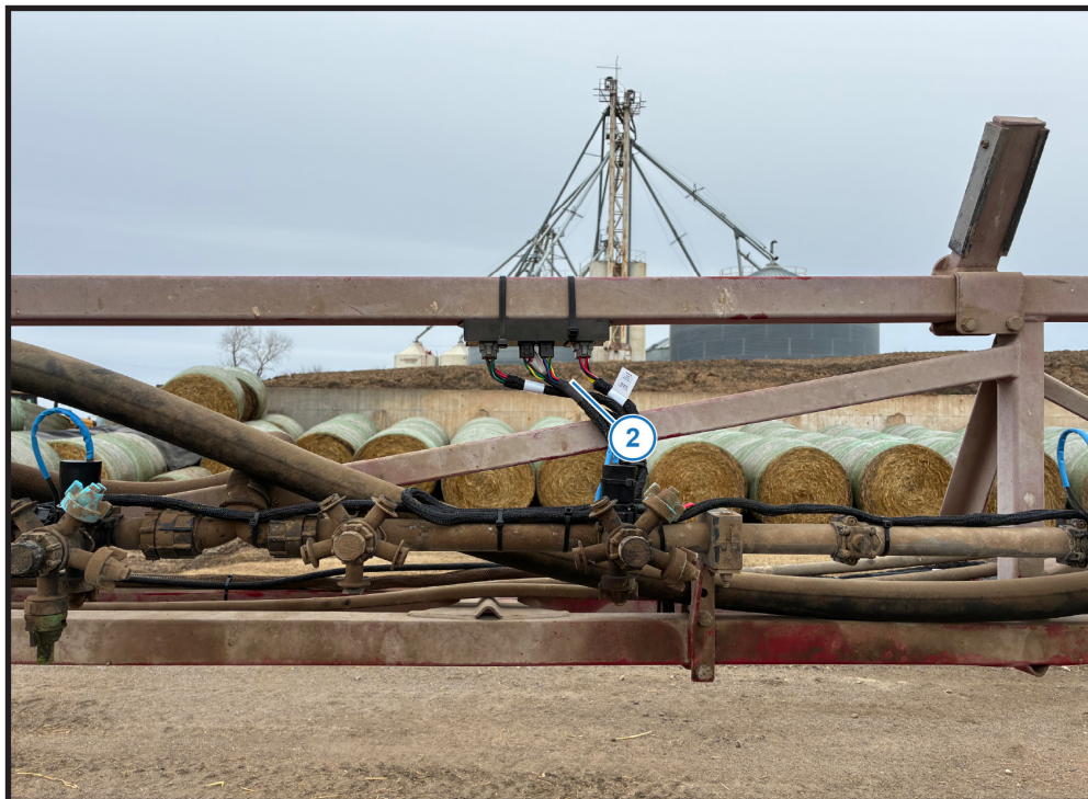
Figure 21: VCM 2 Installation Location
