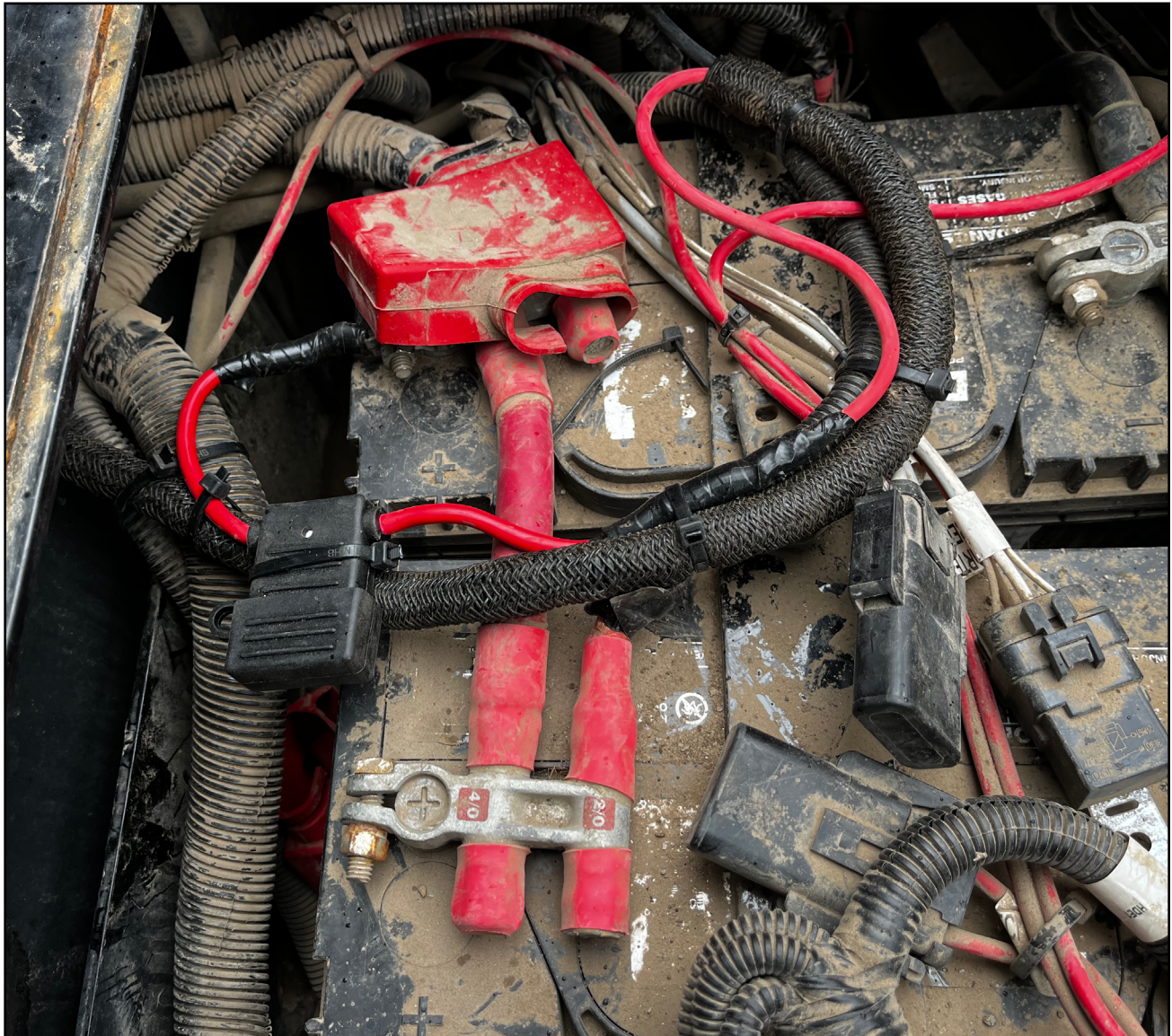
Figure 11: Power Harness and Circuit Breaker
