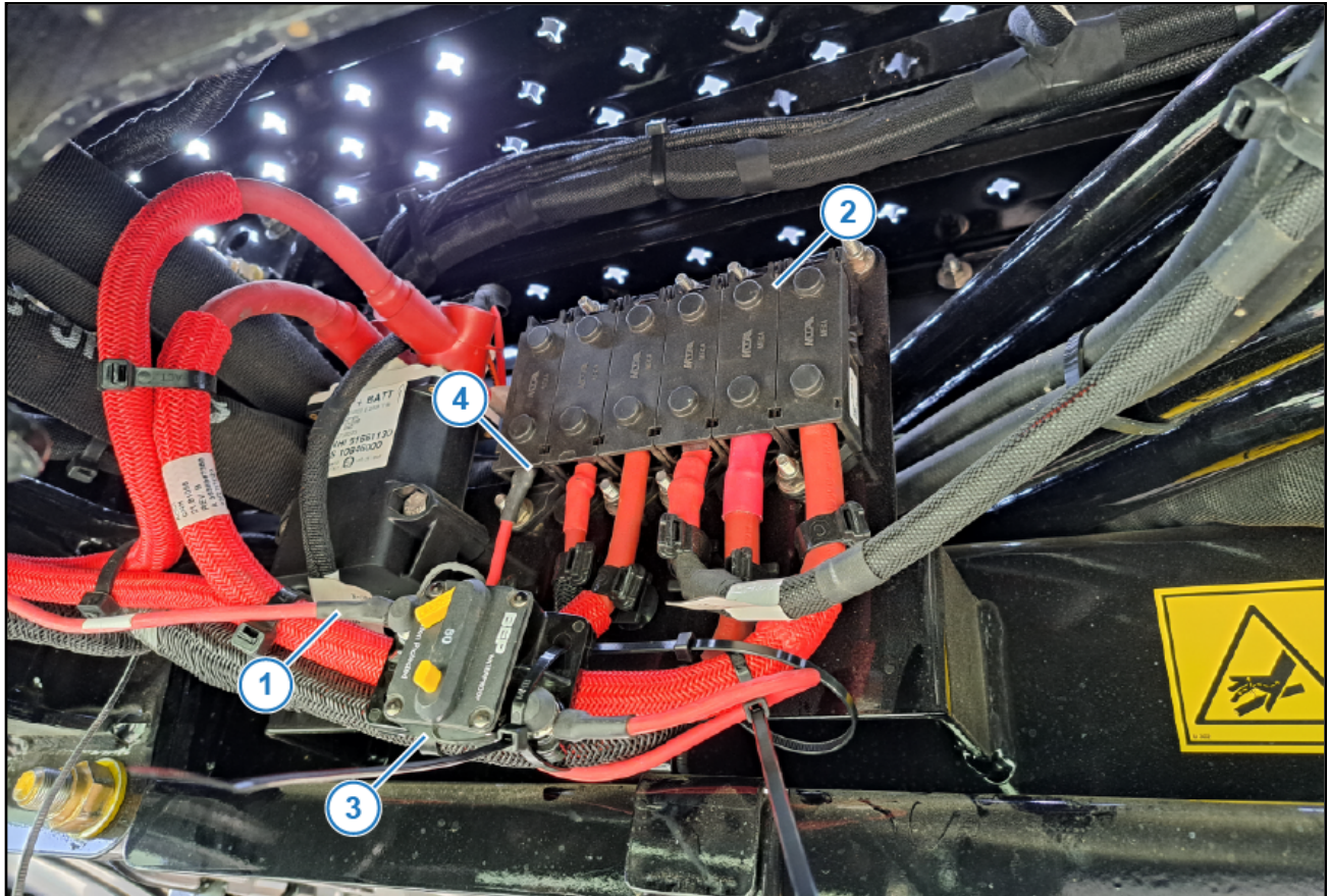
Figure 9: Power Harness Positive Connection
